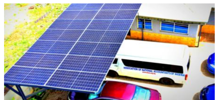
A session of the commissioned solar power system
